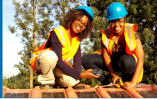
A team installs solar powered roofing tiles on a residential house ©KCIC
