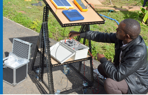
Strathmore Energy Resource Centre staff setting up a solar PV system ©SERC
