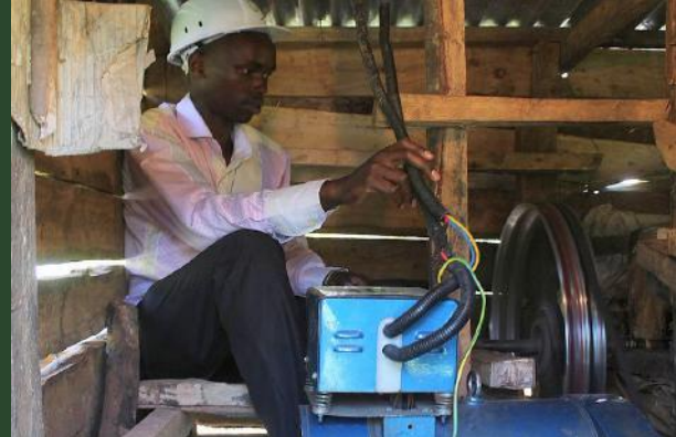
The founder of Magiro Hydro power Plant producing power using fabricated simple motors and old bicycles ©NETFUND
